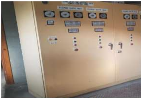
Gate Control Panel
